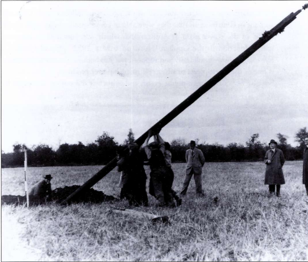
■ Erecting the first pole of the Rural Electrification Scheme at Kilsallaghan, Co. Dublin, on 5 November 1944.
