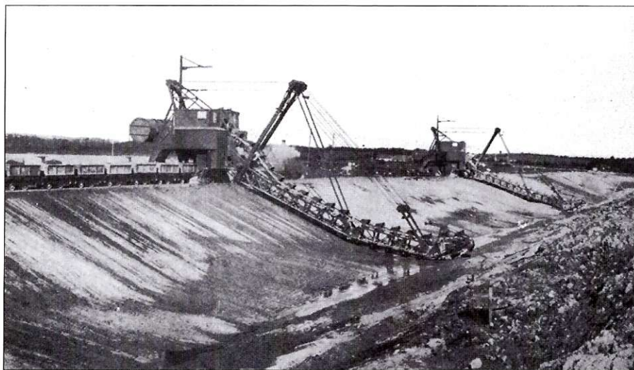
■ Two Buckauer multiple bucket excavators working on the embankment near O'Briensbridge. Source: Siemens Progress on the Shannon Scheme, Number 5, February 1927.
